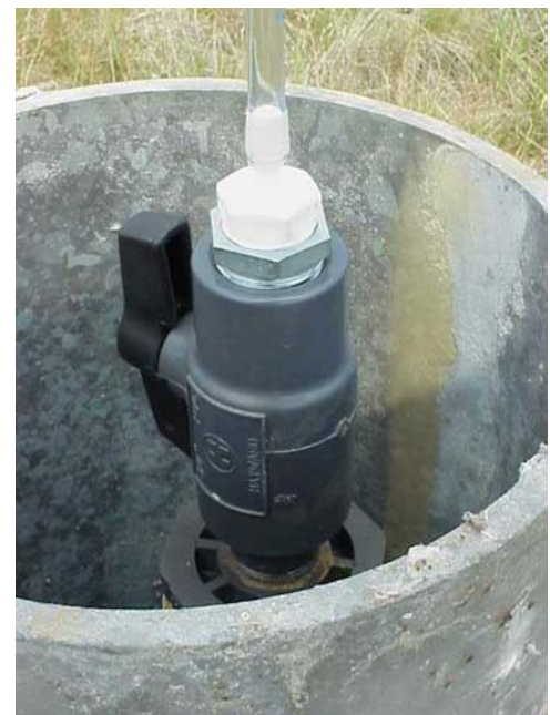
Figure 9.11 Ball Valve for Soil Gas Well, Photographed by C. Van Sciver
