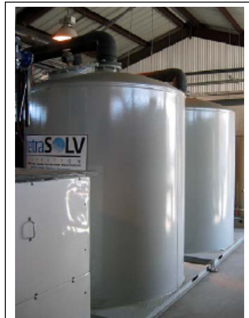
Figure 3. Water Treatment System Carbon Units
