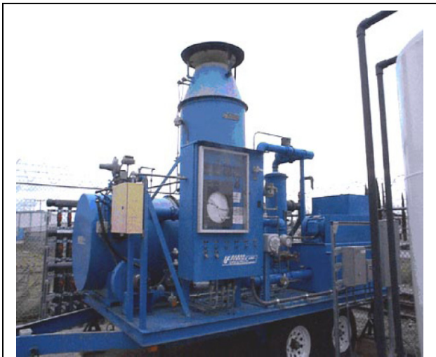
Figure 2. Thermal Oxidation Unit for Treating Vapors Captured by the 1998 SVE System
