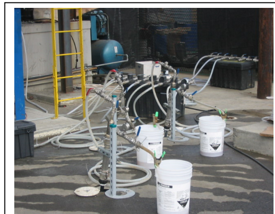
Figure 1. ISCO Application Wells
