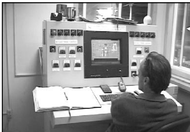
The control room for a 10 ton/day melter system
