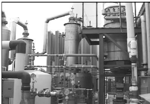
Offgas system with baghouse and two scrubber towers
