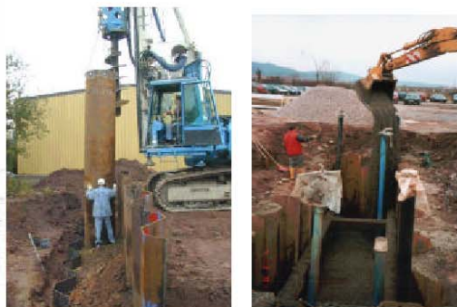
Figure 3 – Right photo: set-up of the vertical drainages using a large diameter borehole construction method; left photo: filling the gate with Fe 0
