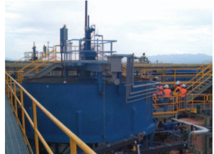
The Sulf-IX™ Plant is designed to remove sulphate from groundwater.
