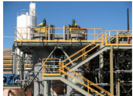
With a design flow rate of more than 25 m 3 /hr, the plant will treat water to produce clean water and a usable gypsum product.
