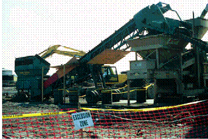
Figure 6.4: Mobile screening and conveying plant (Photograph courtesy of Colin Hills)
