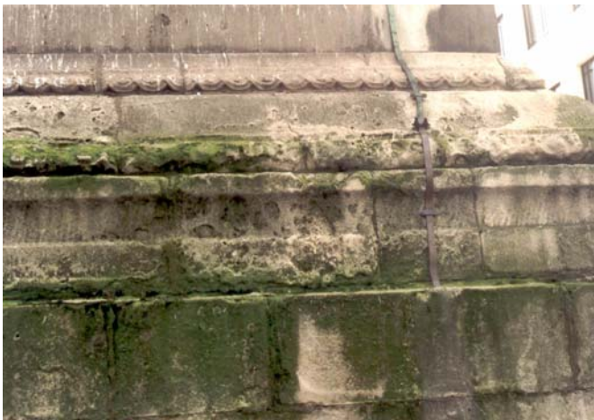
Figure 9.4: Surface degradation of building stone, the London monument. (Photograph courtesy of Paula Carey)
