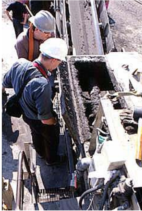
Figure 6.11: Single shaft pugmill mixer with safety screen removed under inspection (Photograph courtesy of The British Cement Association)
