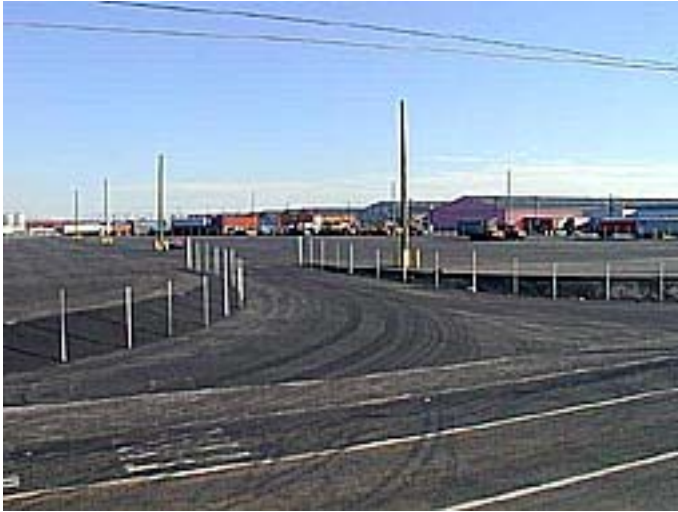
Figure 6.20: Site following completion of wearing course (Photograph courtesy of Portland Cement Association)
