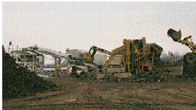
Figure 6.5: Ex-situ operation using mobile plant in centralised manner for treating petroleum-contaminated soils (Photograph courtesy of Keith Bradshaw)
