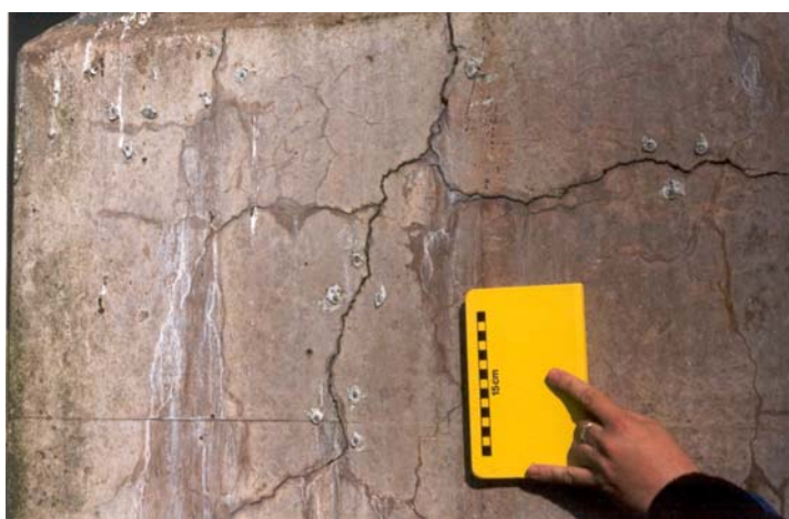
Figure 9.3: Cracking associated with ASR, River Exe Bridges, Exeter, Devon. (Photograph courtesy of Paula Carey)
