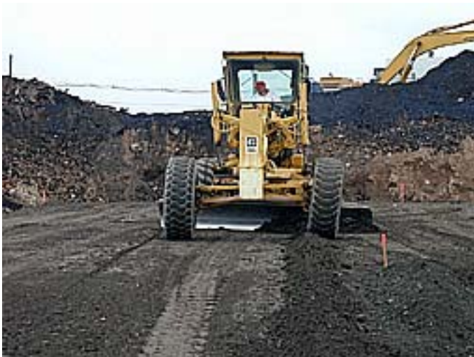
Figure 6.7: Grading of recently S/S creosote contaminated soil (Photograph courtesy of Portland Cement Association)
