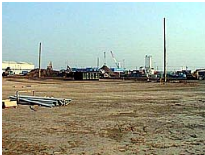
Figure 6.19: Sub-base placed on S/S treated soil (Photograph courtesy of Portland Cement Association)
