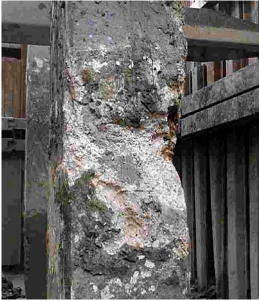
Figure 9.2: Disintegration of a column that has been subjected to thaumasite attack (Photograph courtesy of BRE)
