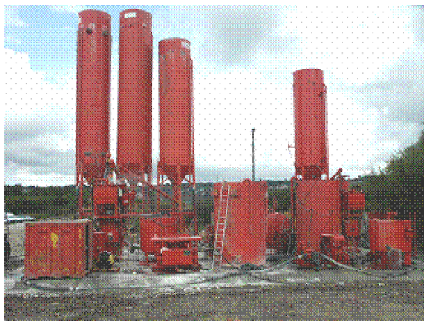
Figure 6.2: Reagent silos/batching equipment for a multi-component binder (Photograph courtesy of Colin Hills)
