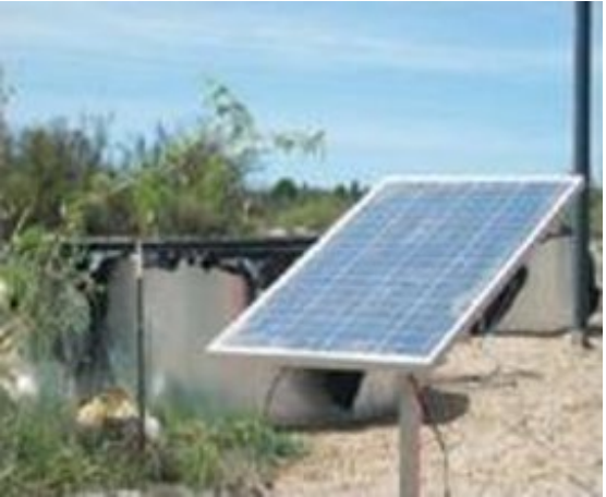
A single PV panel is now used for pumping contaminated perched water from the subsurface for forced evaporation treatment in a brine concentrator.
