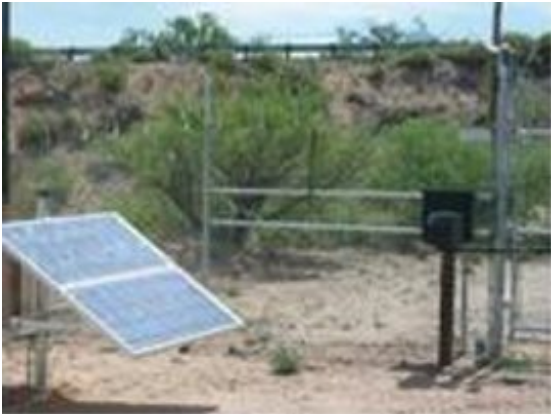
Additional PV arrays provide electricity for wetlands area lighting, motion detection, security cameras, and gate controls.
