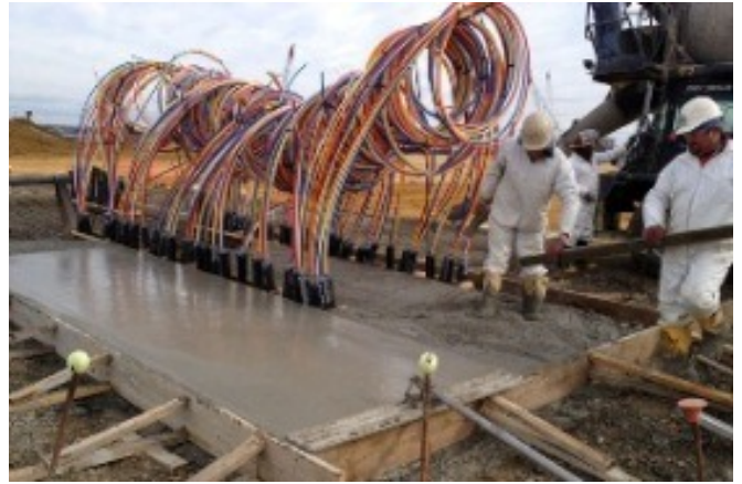
Ozone Sparge System Installation: In 2011, an ozone sparge system was installed to accelerate removal of contaminant vapors from groundwater in two contaminant source areas.
