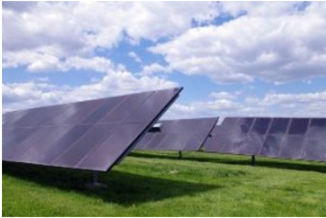
PV Arrays: Each PV array was installed on concrete footers designed to accommodate the landfill cover system's operation and maintenance requirements.
