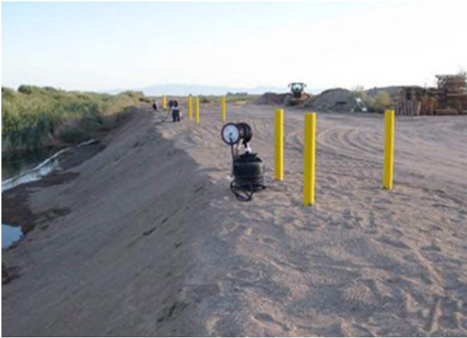
Product Recovery Pumps: Free product is recovered through use of a pneumatic skimmer pump in each of eight wells. Along the eastern edge of the irrigation drainage canal adjacent to the site, a 140-foot-long interceptor pipe housing a product boom was installed and plumbed into the recovery system to capture additional free product.
