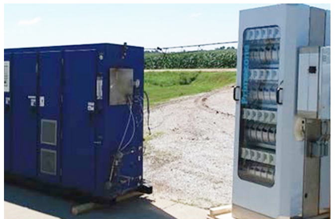
AOP Upgrade: Replacement of the ozone generator operating since 2007 (shown on left) with a technologically advanced generator (on right) was a key component of the 2019 AOP upgrade.
