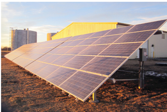
Solar Power: One of the site's three 25-kW PV arrays operates near the main treatment plant.
