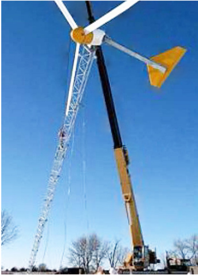
Wind Turbine: The 10 kW wind turbine was installed in early 2004 at a location next to the site's groundwater recirculation well. Relevant wind conditions included a speed of 6.5 meters/second, shear exponent of 0.27 and turbulence intensity of 0.17-0.21.
