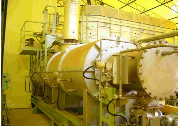
Thermal Desorption (Screw Conveyor)
