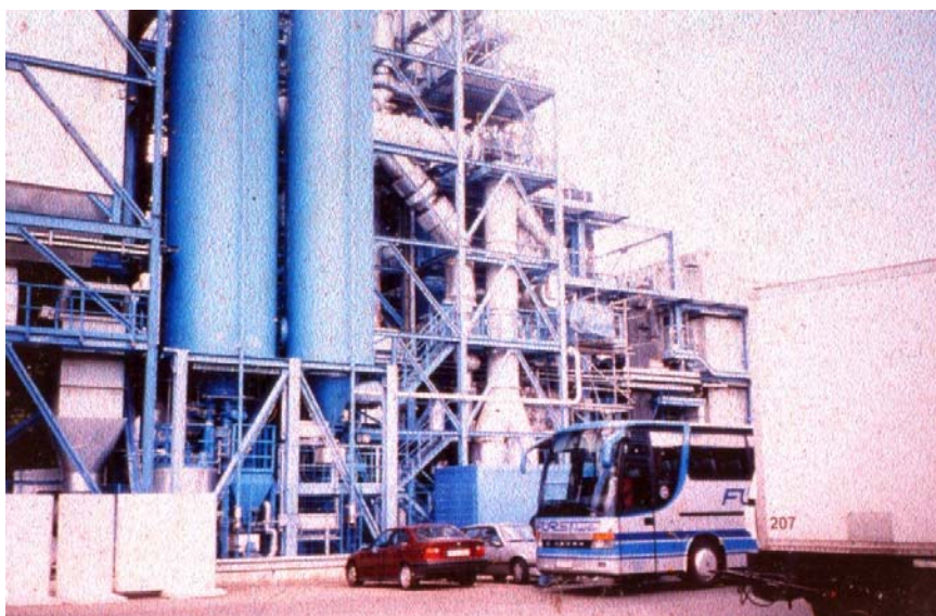
Figure 8: View of the Boran Thermal Treatment Plant, Berlin - NATO pilot study 1996 (BARDOS, 2002)
