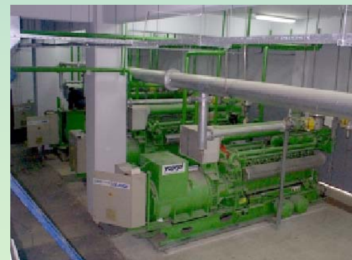
İstanbul- Kemerburgaz Landfill Gas Facility
