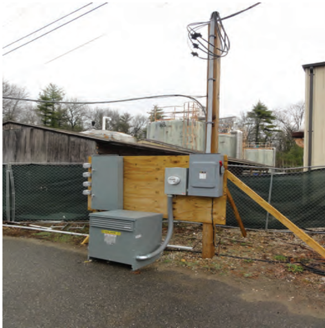
TEMPORARY POWER SERVICE INSTALLED AT SITE 8
