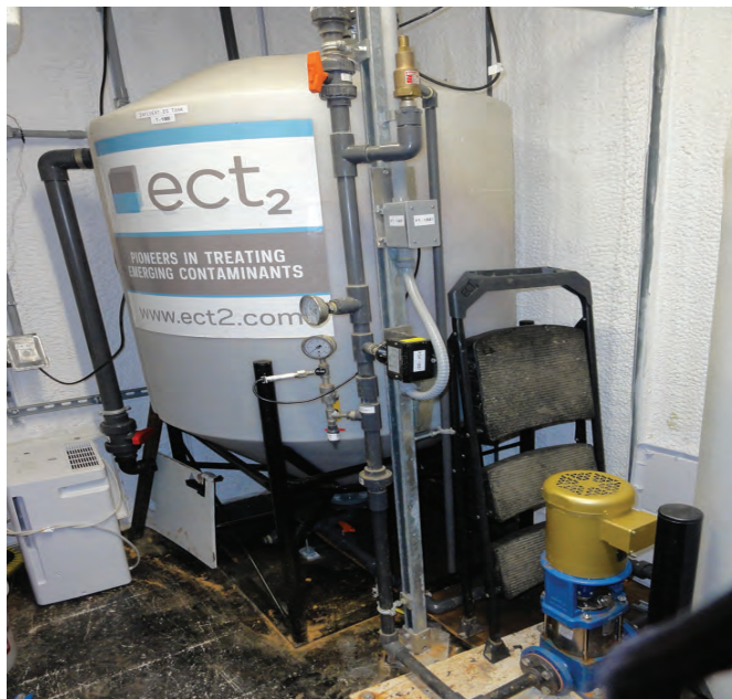
EQUALIZATION TANK AND FEED PUMP
