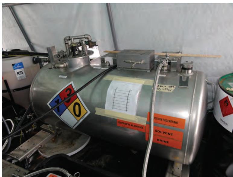
REGENERANT RETURN TANK
