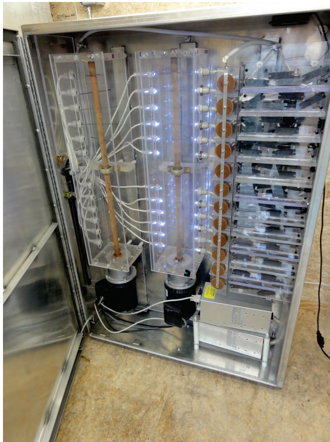
POWER SUPPLIES IN OPERATION
