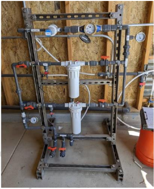
Figure 4. Pre-filtration skid in pilot building
