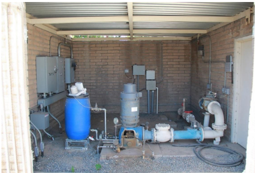
Figure 2. OCWD Bessie well facilities
