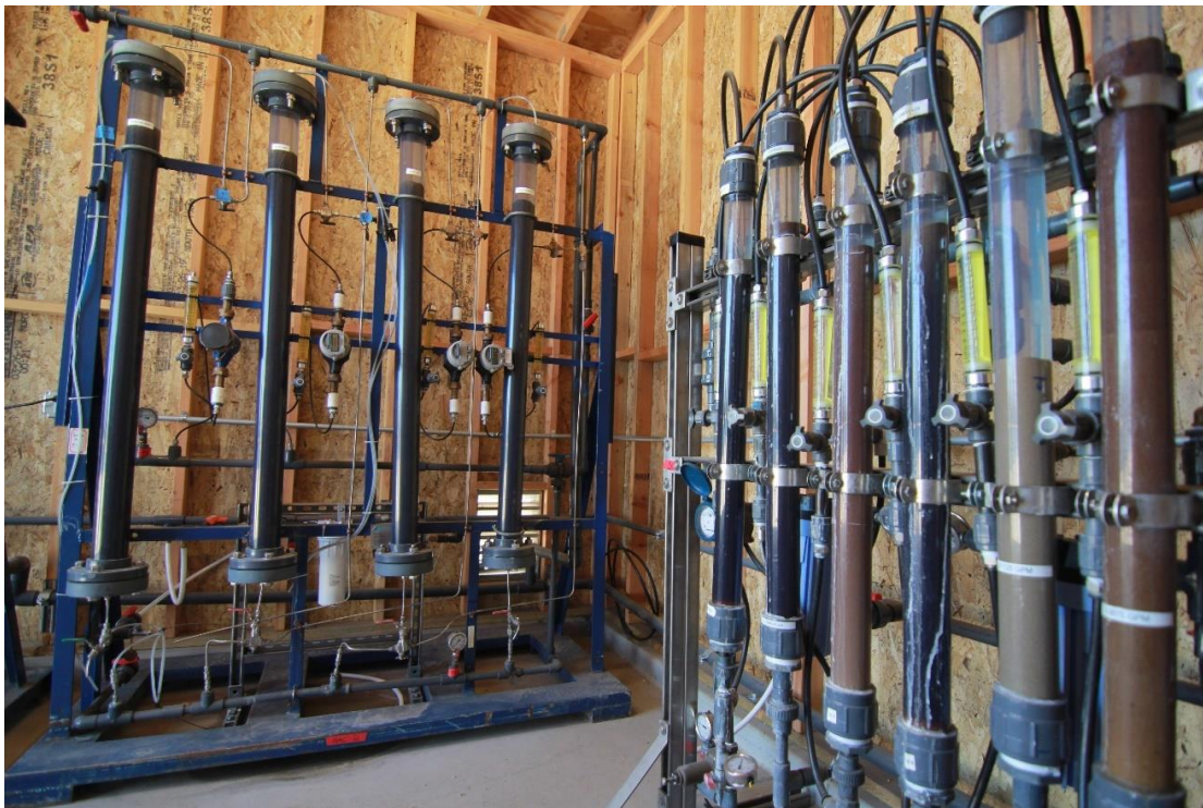
Figure 5. GAC skids (left, partial view of four of eight columns) and IX/alternative adsorbent skid (right) placement in pilot building
