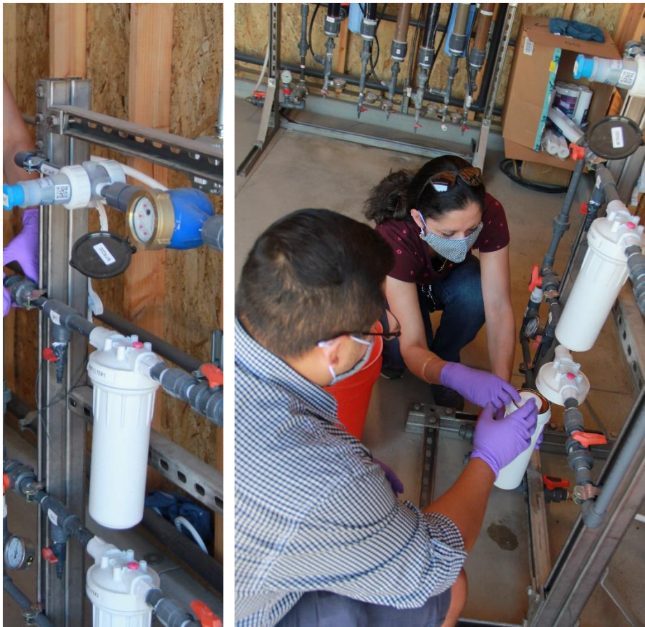
Figure 9. Influent cartridge filters (left) and cartridge filter replacement (right)
