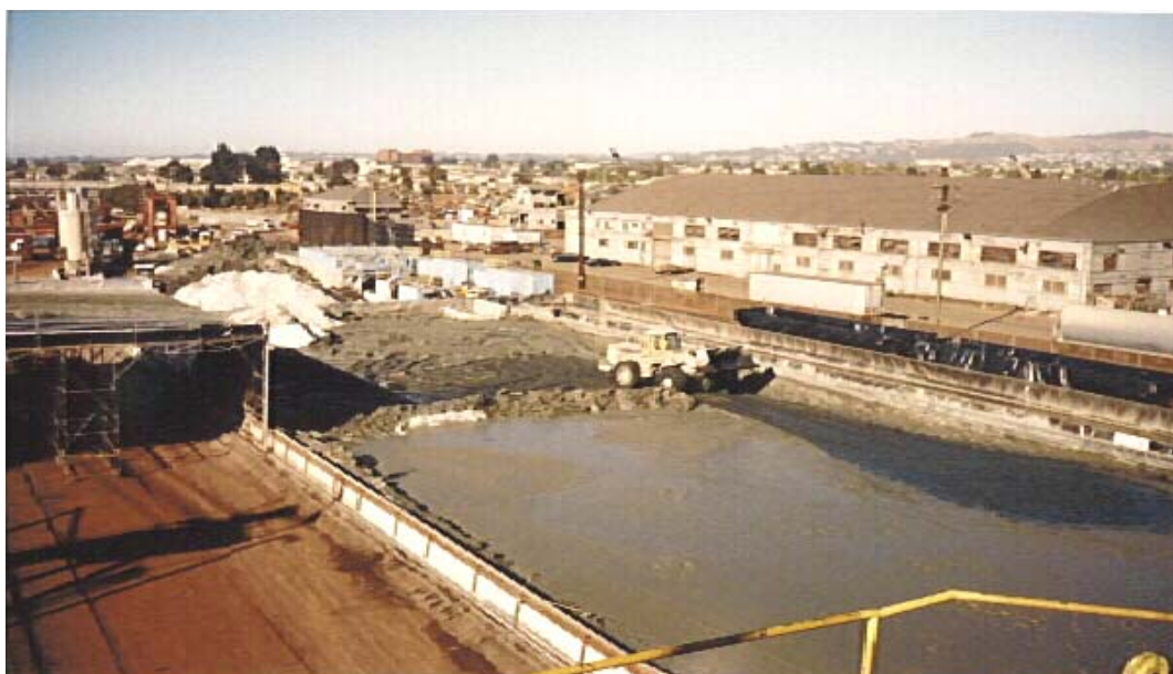
Figure 4-5. Dewatering and Pretreatment Facility for Dredged Sediment
