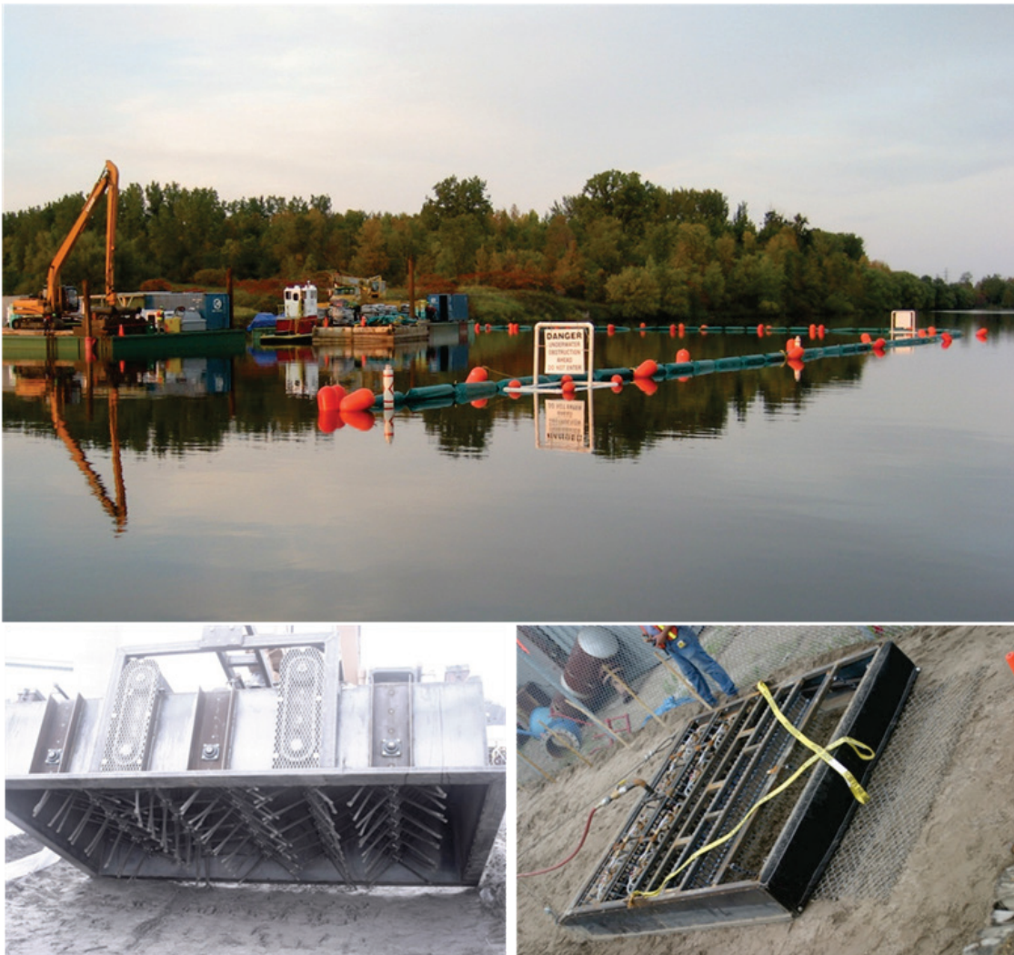
Figure 3. Activated carbon (AC) deployment for the Grasse River pilot study in 2006. Two different devices used to deploy AC included a steel box with an enclosed tiller (bottom left) and a sled with injection tines (bottom right). (Modified and reprinted with permission from Beckingham and Ghosh 2011, 10569. Copyright 2011 American Chemical Society.)
