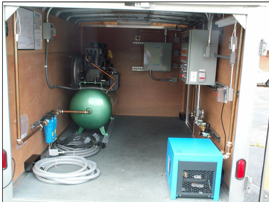
Figure 5-19. Inside of Trailer #1 which houses the controls and air supply system.
