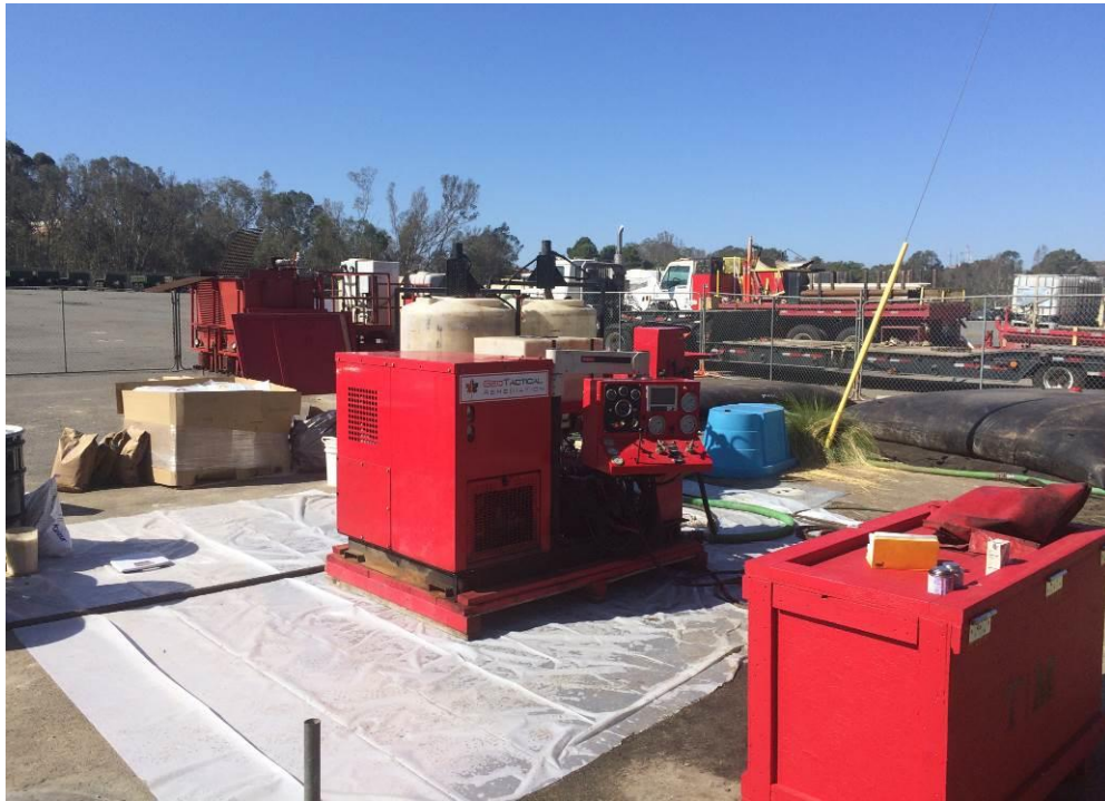
Photo 5 – EFI2000 Mixing and Pumping Unit with Ancillaries
