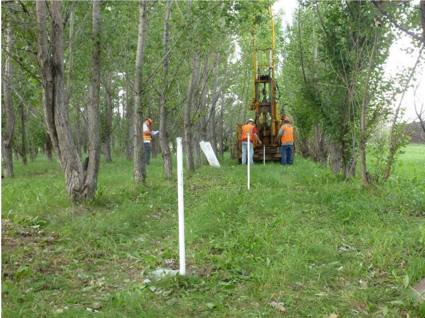
Figure 5-12: Temporary injection well installation and tree spacing at Grand Forks AFB TU504.
