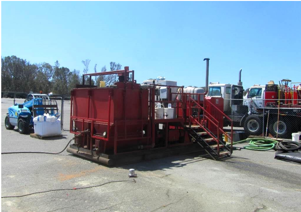
Photo 1 – EF9300 Fracturing Unit with Ancillaries
