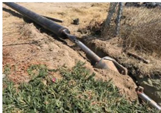
Figure 22. Well installation Reaming tool attached to 12-inch diameter steel well materials prior to pullback
