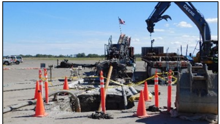
AF contractors conduct horizontal well drilling at the former Galena FOL. Photo Courtesy: AF Contractor
