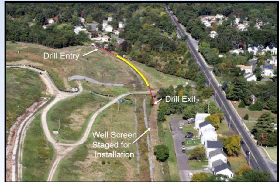
Horizontal Hydraulic Control Well for Landfill Leachate Containment
