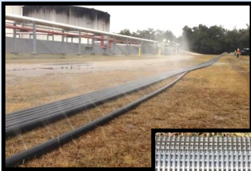
Water being pumped through horizontal remediation well to demonstrate uniform flow through well screen
